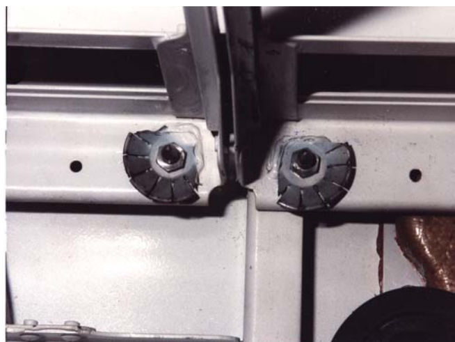
Figure 6-5. EMI Bonding Washers in Avionics Bay
